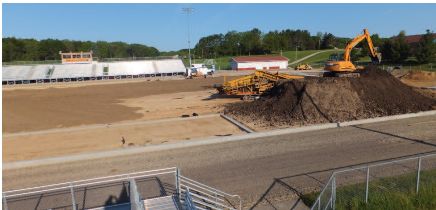
Construction of Verona Area High School's stadium field will be featured during the afternoon sports field manager's tour
