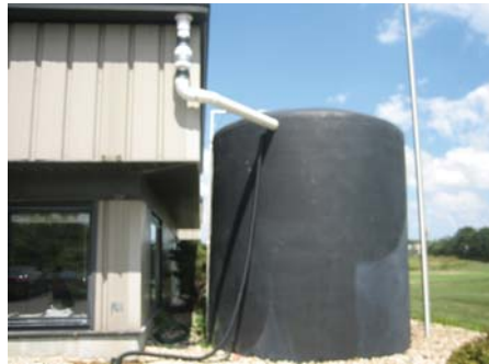
(1) Aboveground tank located on the Southeast corner of the building. Visible are the water collection conduit and overflow vent.
