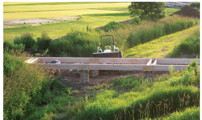
Forms were constructed for pouring the concrete piers and deck support beams
