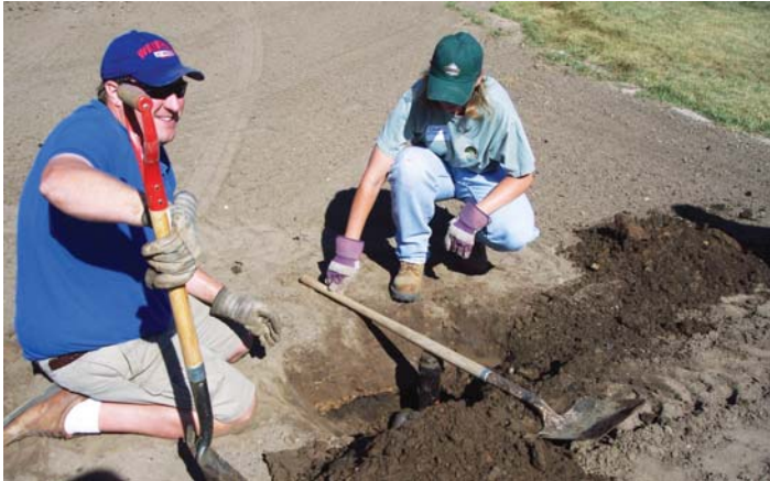
Brett Grams and Dena DiVincenzo from Waupaca Sands and Solutions doing some irrigation work on the new field.
