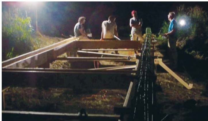
The crew working through the night to tie reinforcing steel bar before the concrete arrives the next morning
