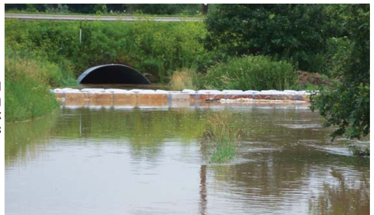
The flood that occurred the day after pouring the piers and deck support beams
