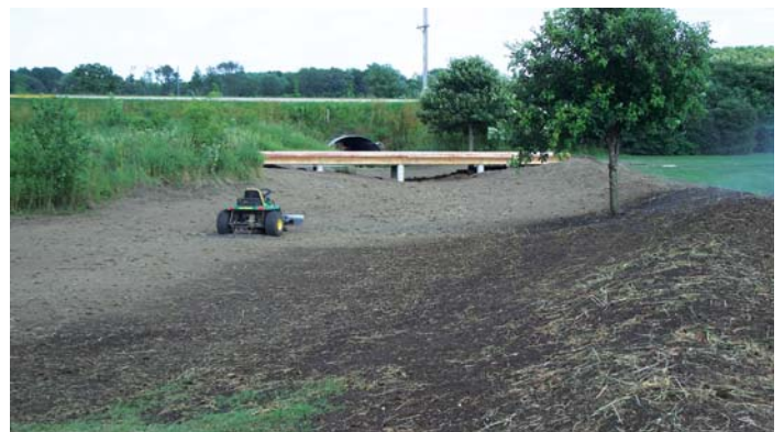
The new drainage swale will move floodwaters past the Noer Facility more efficiently
