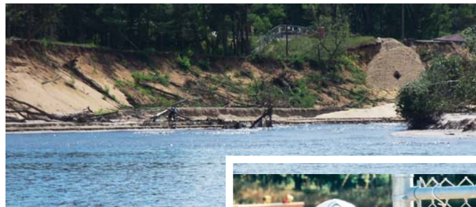
This breach that emptied Lake Delton was caused by the same rain event that devastated Kaminski Park, site of the Extreme Makeover.
