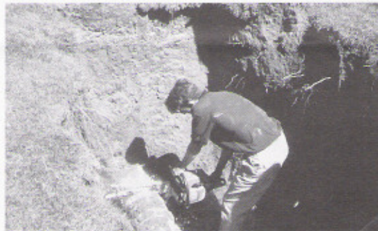
A chain saw was used to repair this 12-inch mainline after a land shift.
