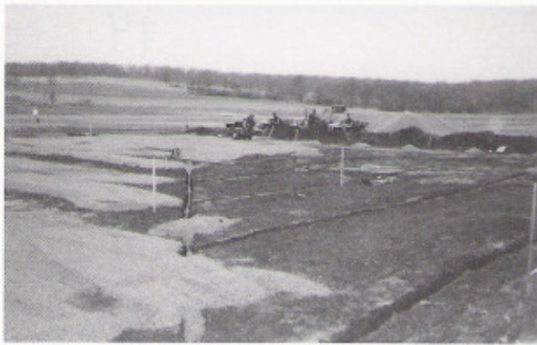
We were racing the gun to try to get the drainage tile covered before a thunderstorm broke this day.
