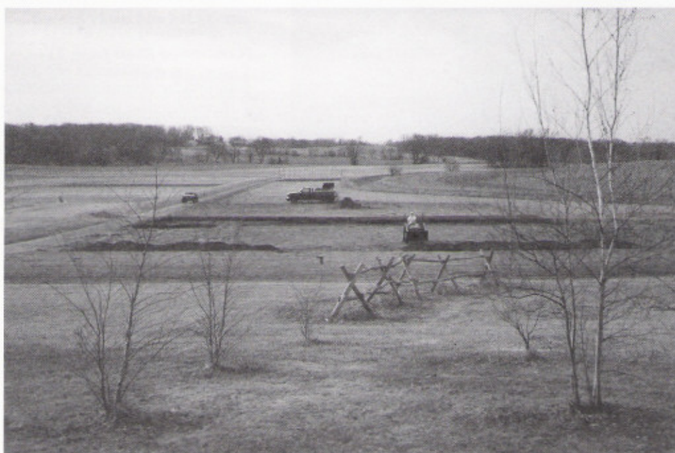
Hauling away the old sod and starting to build the push-up green.
