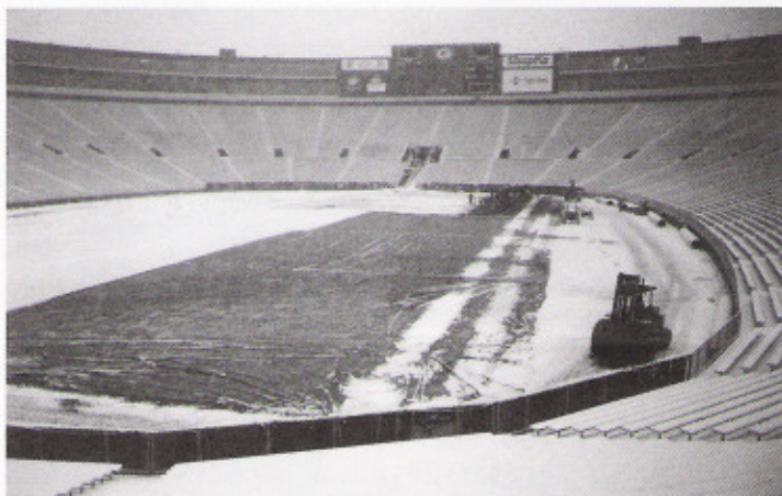
The sod has yet to be laid where the tarp is located.
